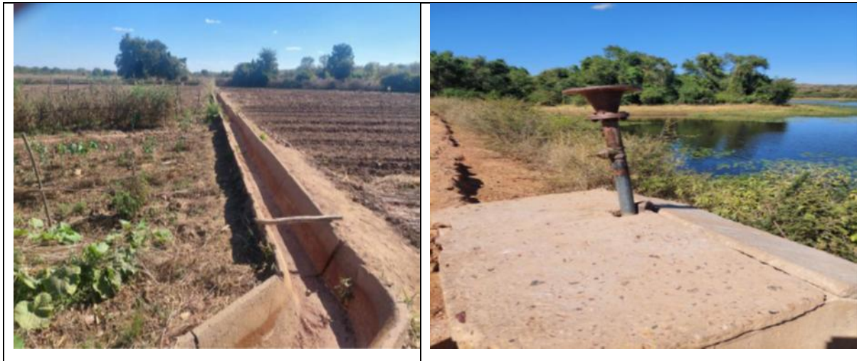
Plate 6: Facilities at Takavinga Irrigation Scheme
