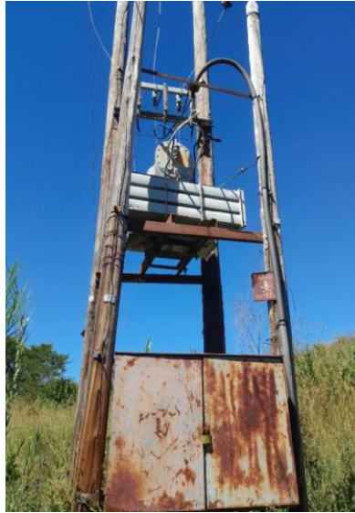
Plate 2: 250kVA Transformer at Athlone Irrigation Scheme
